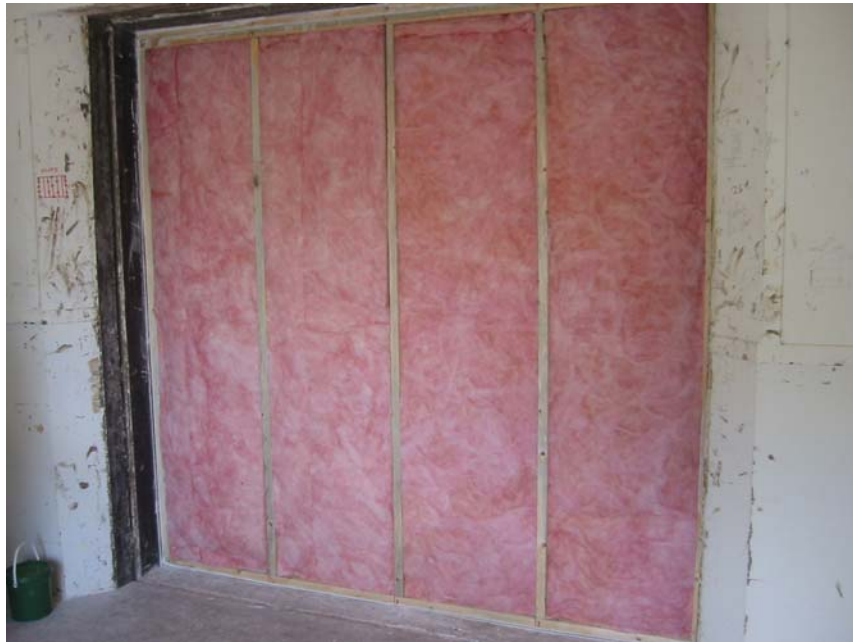
Figure 2: Framing and insulation prior installation of sheeting (viewed from source room side).
